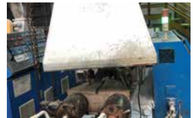
Exhaust gas treatment device in a workshop
